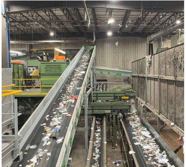
Conveyor lines transporting recyclables at the Syracuse WMRA Materials Recovery Facility in Liverpool, NY.
