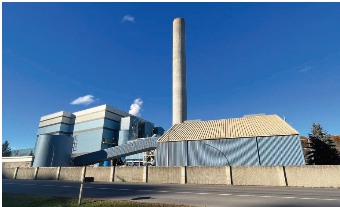
The Waste-to-Energy Facility on Rock Cut Road in Jamesville converts trash into enough electricity to power roughly 30,000 households in Onondaga County.
