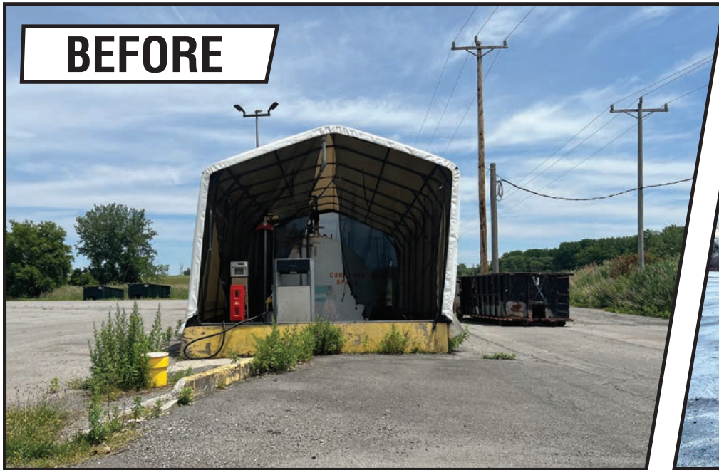
Before demolition, an aging fuel station stood on the edge of the Ley Creek Transfer Station property.
