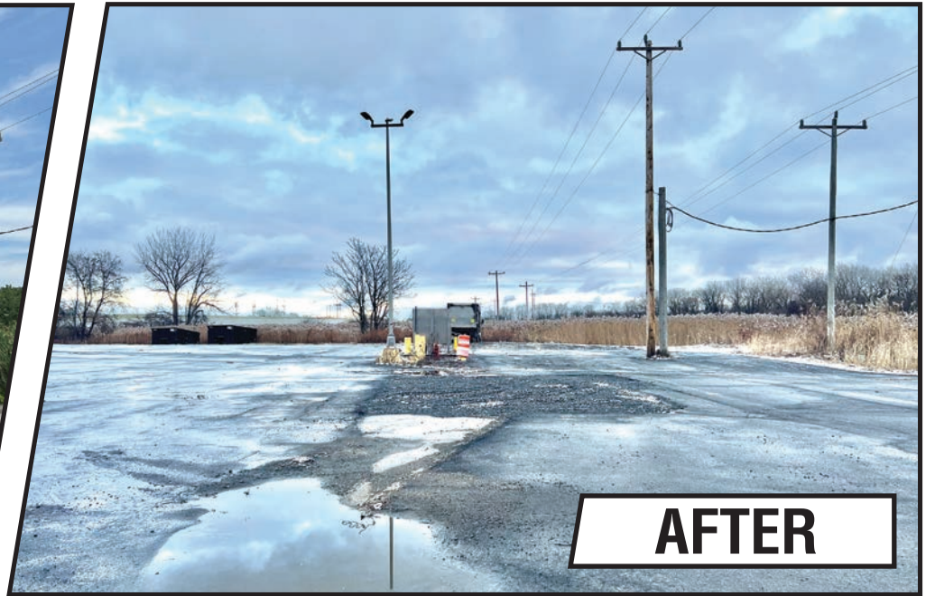
After demolition, the fuel station was among the first structures removed to make way for a modern facility.
