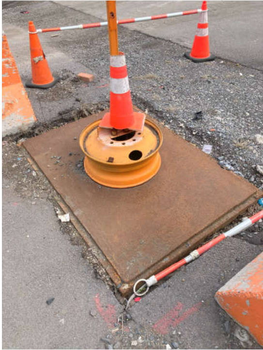
Photo 4: North Site Area, electrical vault cover
