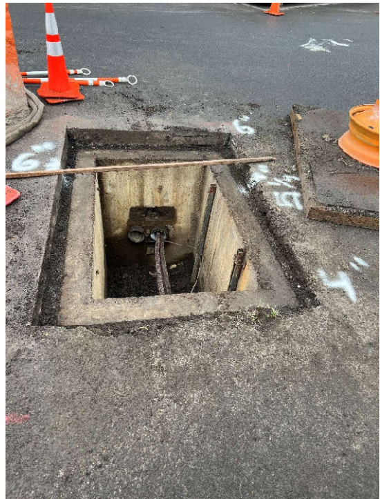
Photo 5: North Site Area, electrical vault
