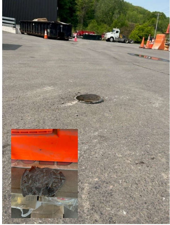
Photo 2: North Site Area: water riser (insert: damaged water riser cover)
