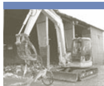
Heavy equipment is used to sort out materials. Last year, the workers recovered more than 4,000 tons of metal and corrugated cardboard.
